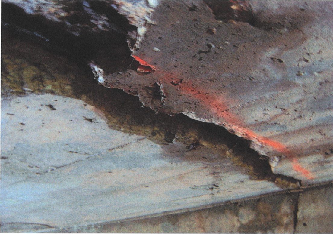
1" crack in bottom of top slab
