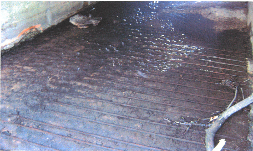
Bottom slab eroded
