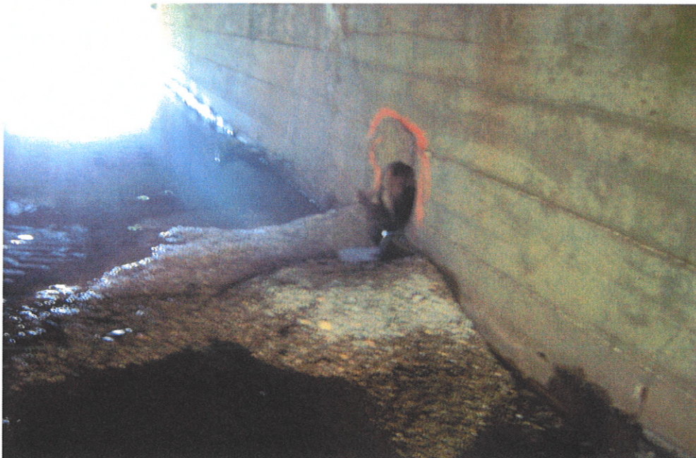
Pipe carrying storm water has failed, allowing rock and sediment to filter in, creating a void in the roadway above.
