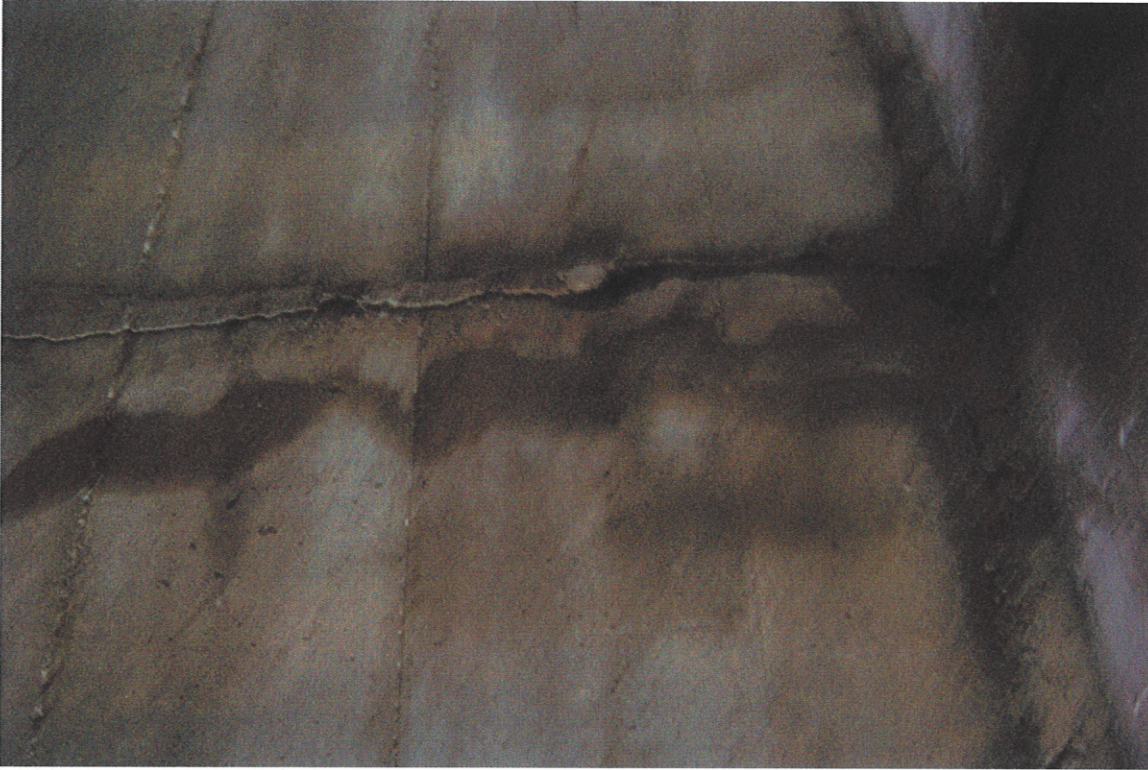
1/4" - 1/2" crack in back wall (typical)
